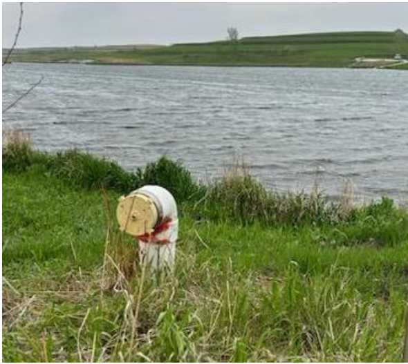
Dry hydrant at Young Pond, Grove Township
